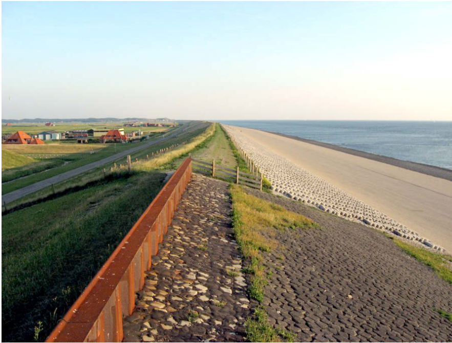
Figure 10.30: Additional sheet piling at crest of dike, Hondsbossche and Pettemer sea defence. From Wikipedia, uploaded in 2005 ('Credits' on page 579).
