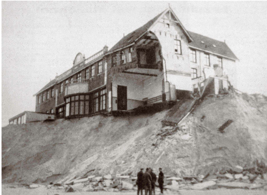
Figure 10.6: Historical photo of damage to a hotel at Schiermonnikoog due to dune erosion, circa 1923. From Rijkswaterstaat ('Credits' on page 579).
