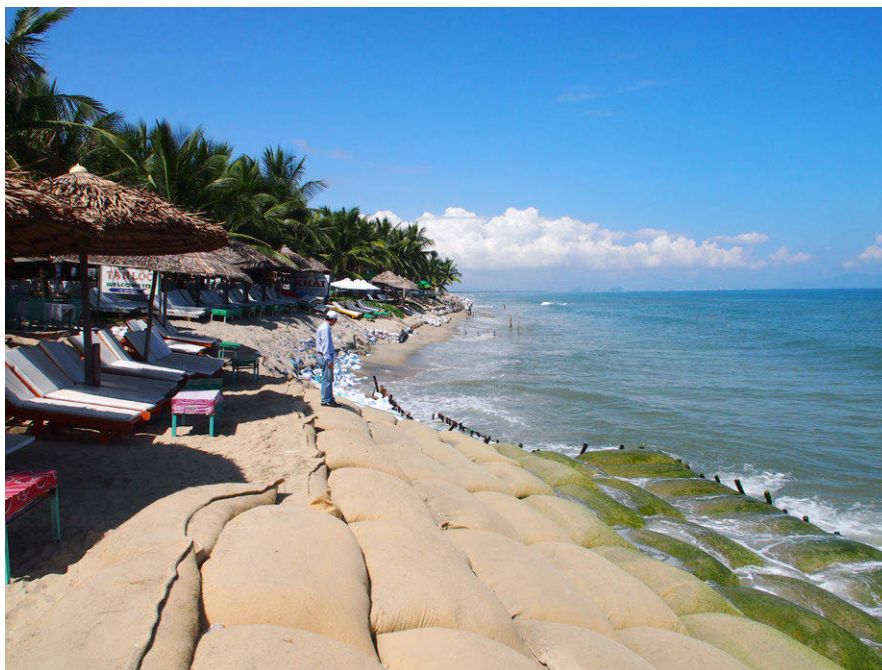
Figure 10.21: Cross-shore and longshore damage to an incorrectly applied revetment, Cua Dai beach, Hoi An, Vietnam, around 2016. Photo by Marcel J.F. Stive ('Credits' on page 579).
