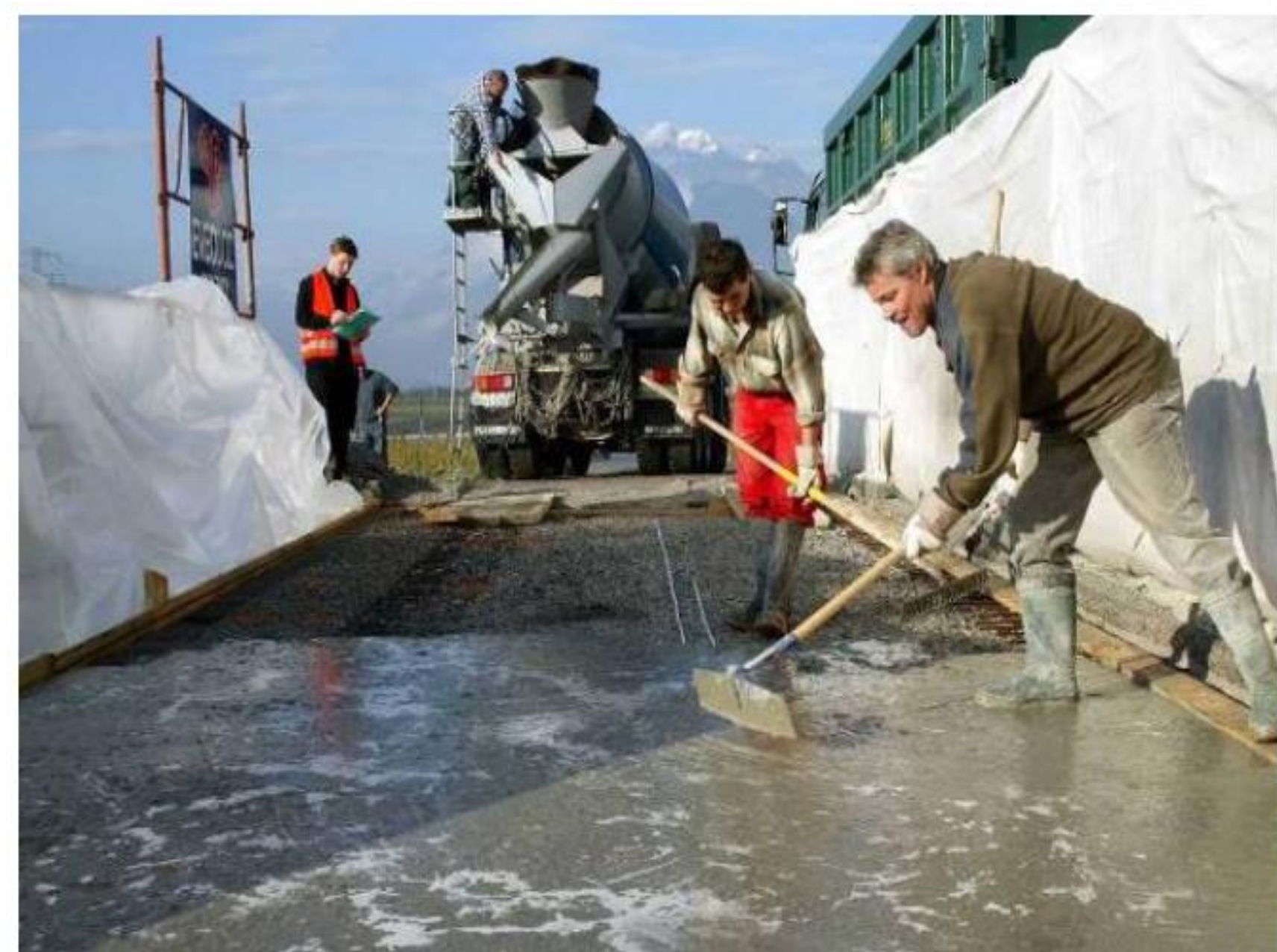
Damaged concrete bridge strengthened by new concrete
