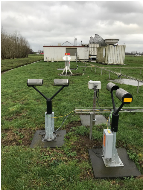
Disdrometers in Cabauw for measuring raindrop size distributions
