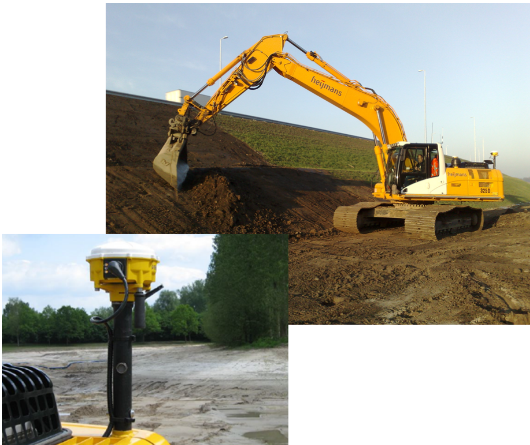
Fig. 9: Excavator in the process of constructing a motorway embankment, as an example of machine guidance. GPS-RTK provides accurate real-time position information (note the two GPS-antennas on the back of the engine). Image courtesy of Heijmans .
