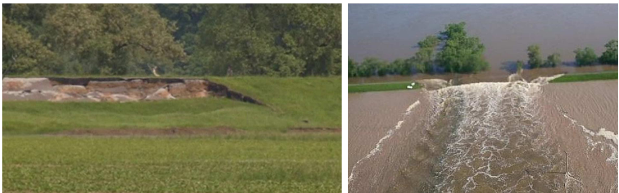
Figure 1: Levee Failure (Breitenhagen, Germany, June 2013). Left: initial stage of the failure process, probable cause was instability. Right: breach in progress.
