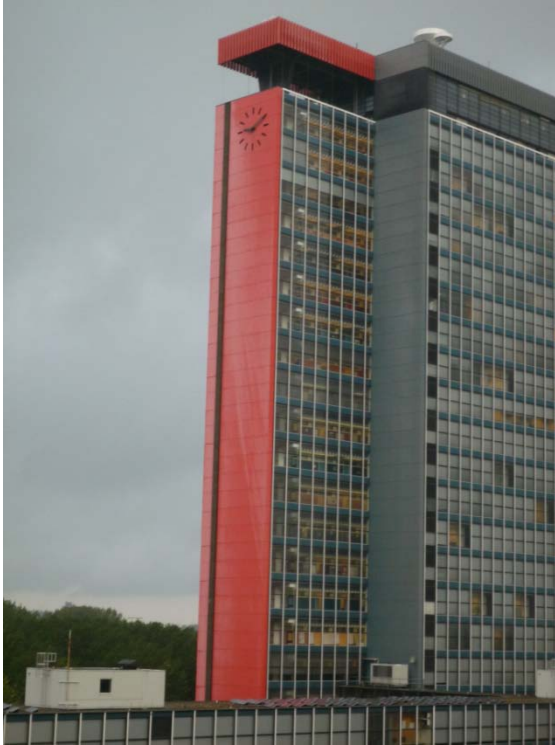
Figure 23: Effect of rain and wind on side of EWI building
