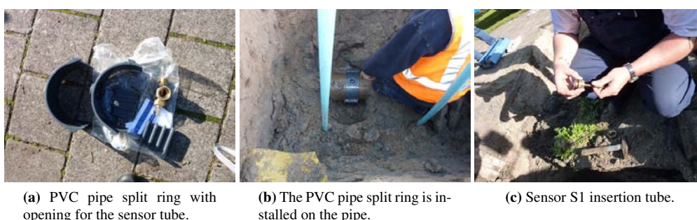
Figure A.13: PVC pipe split ring with opening for the sensor tube.
