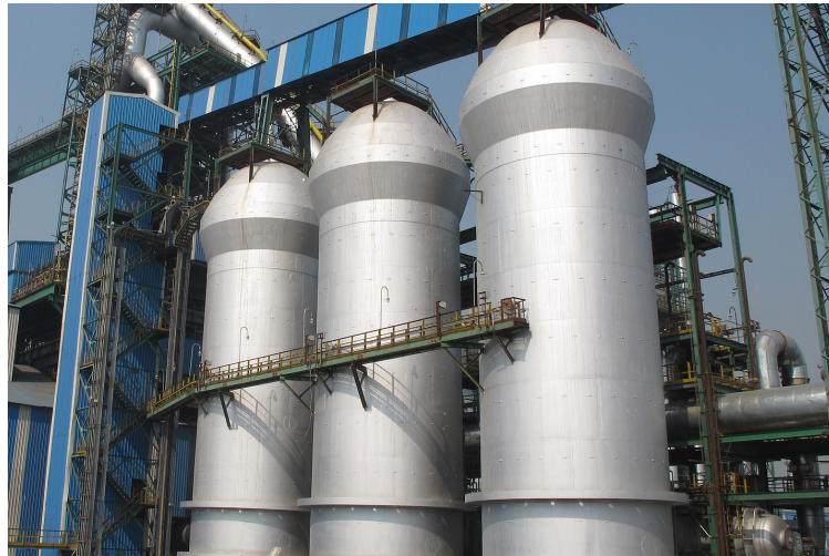
Figure 1: Hot blast stove supplying hot air in the steel making process.
