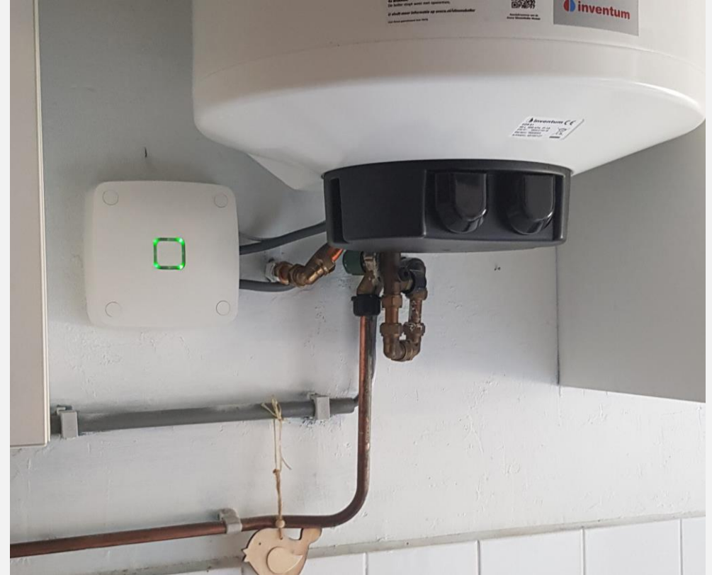
Remotely activate a pool of 10k + electrical boilers
