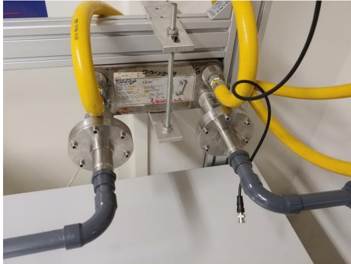
Figure B.3: Heat exchanger coupled with the loop and 2 tubes which contain the cooling water
