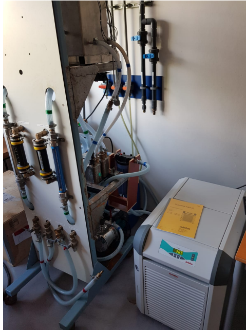
Figure 3.7: Picture of the two cooling installation used in both Scrooge setups. The left installation is the secondary loop, which is connected to the internal cooling system of the building. The right installation is the disconnected cooling installation, which regulates itself.
