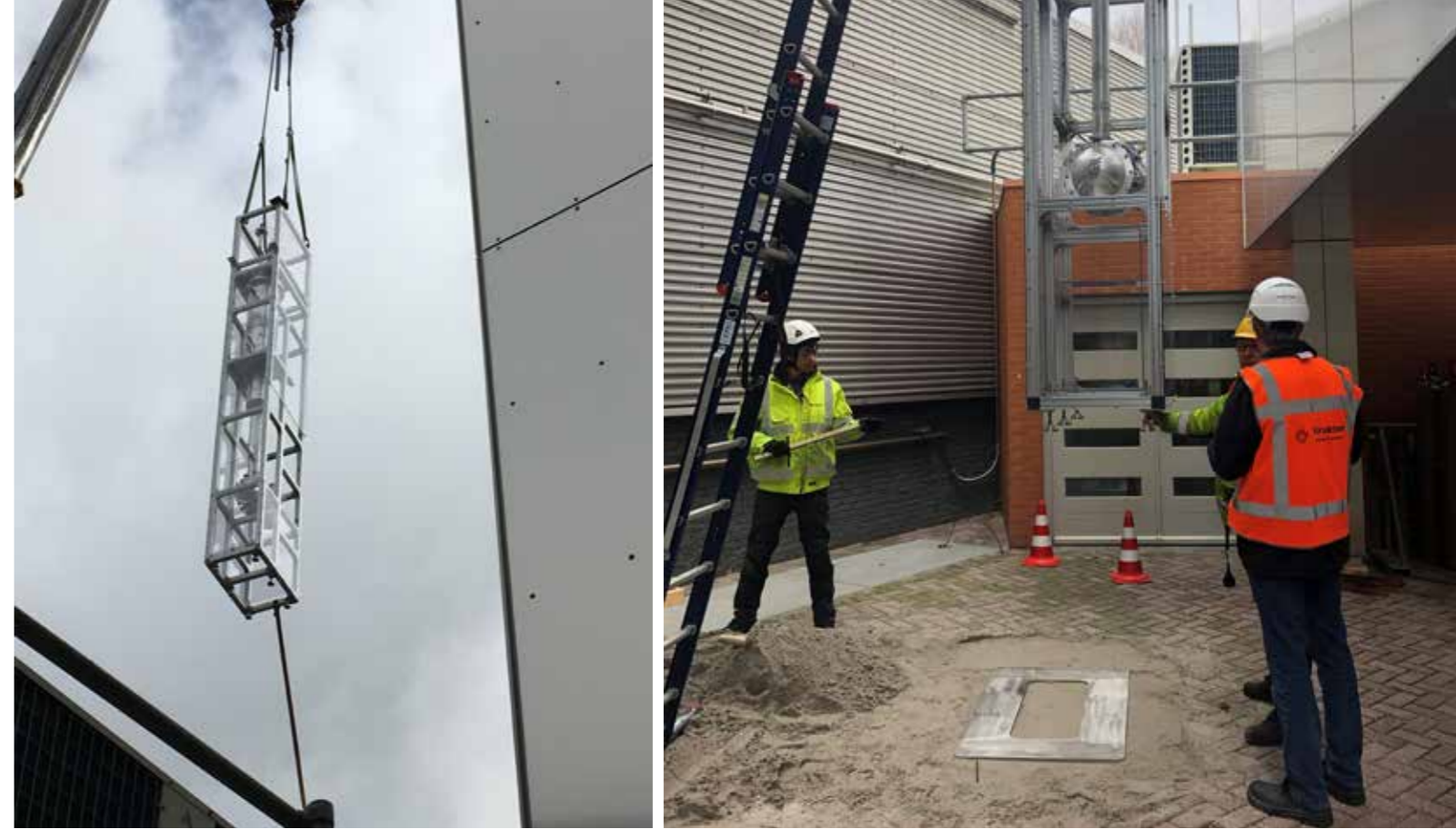
Photos: The arrival of the mock-up of the In-Pool Assembly (IPA) from Korea.
