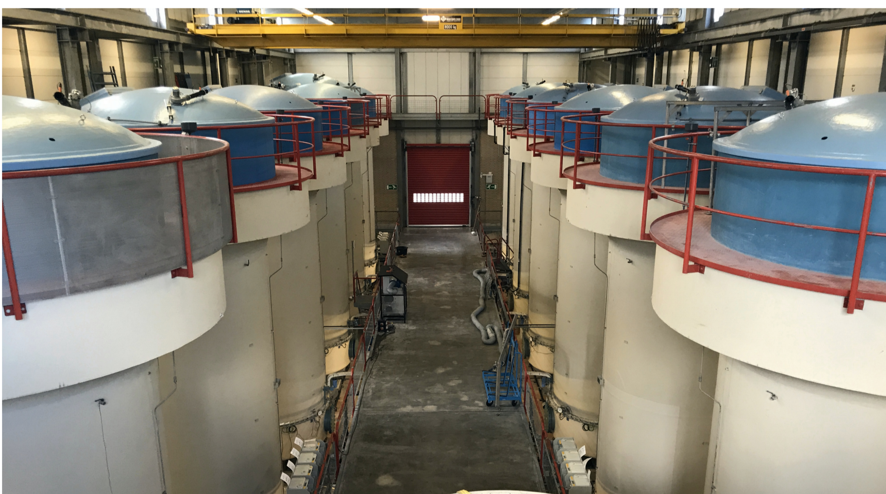
Fig. 2: Full-scale pellet-softening reactors located at Waternet (Amsterdam, the Netherlands). The unit consists of 12 reactors with a column diameter 3 meter
