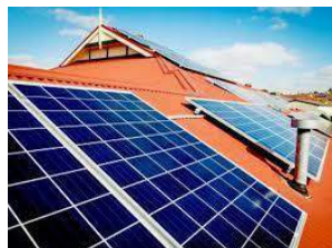
Rooftop system ~2-10 kWp
