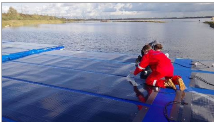
Solar foils on floating system (project Solar@Sea, NL)
