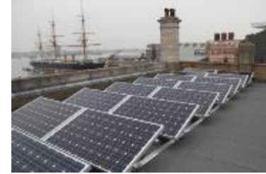
Built-Added Photovoltaics (BAPV)
