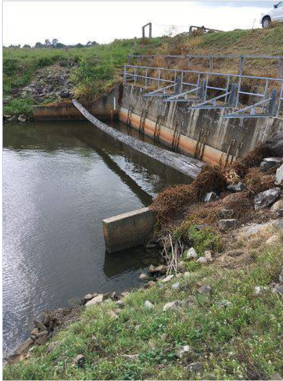
Figure C.1: Overview of the outlet walls of the Swan Creek Floodgate towards the Clarence River.
