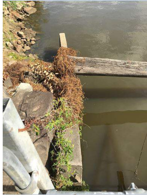
Figure C.2: Current state of the outlet wall of the Floodgate. It is clearly visible that the outlet wall is tilted.
