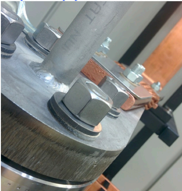
Electrical connection to heated section
