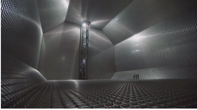
Figure 1. The interior of a Mark III LNG membrane tank.
