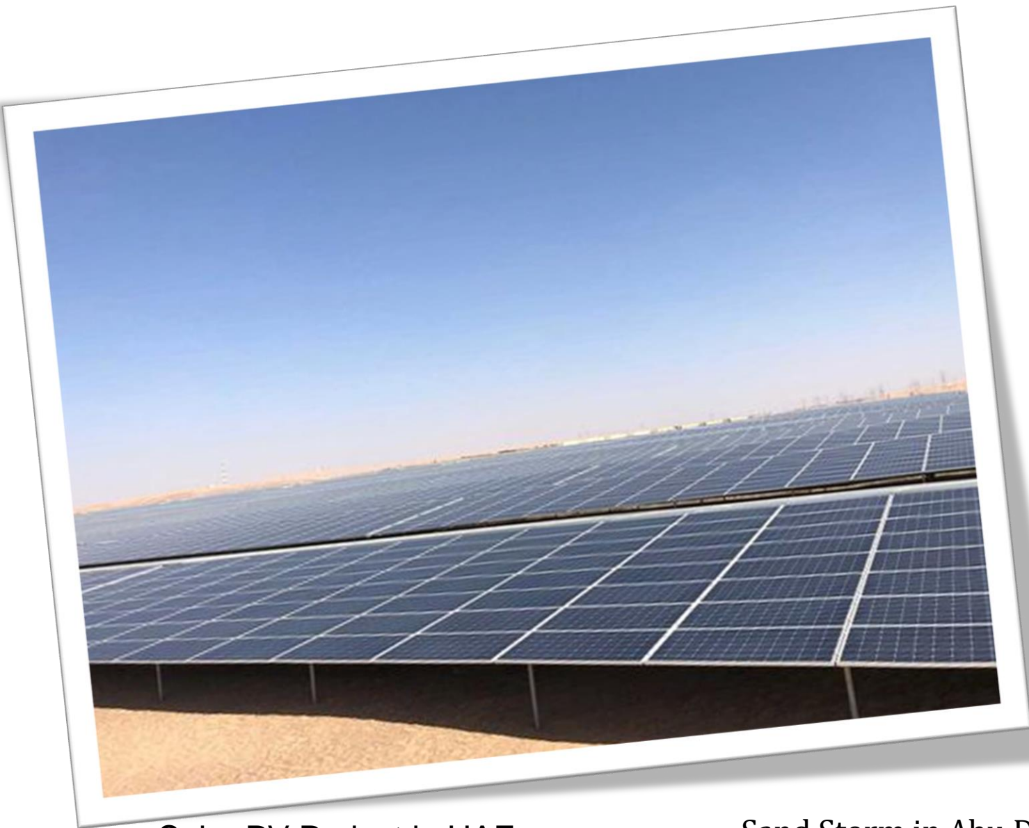
Solar PV Project in UAE
