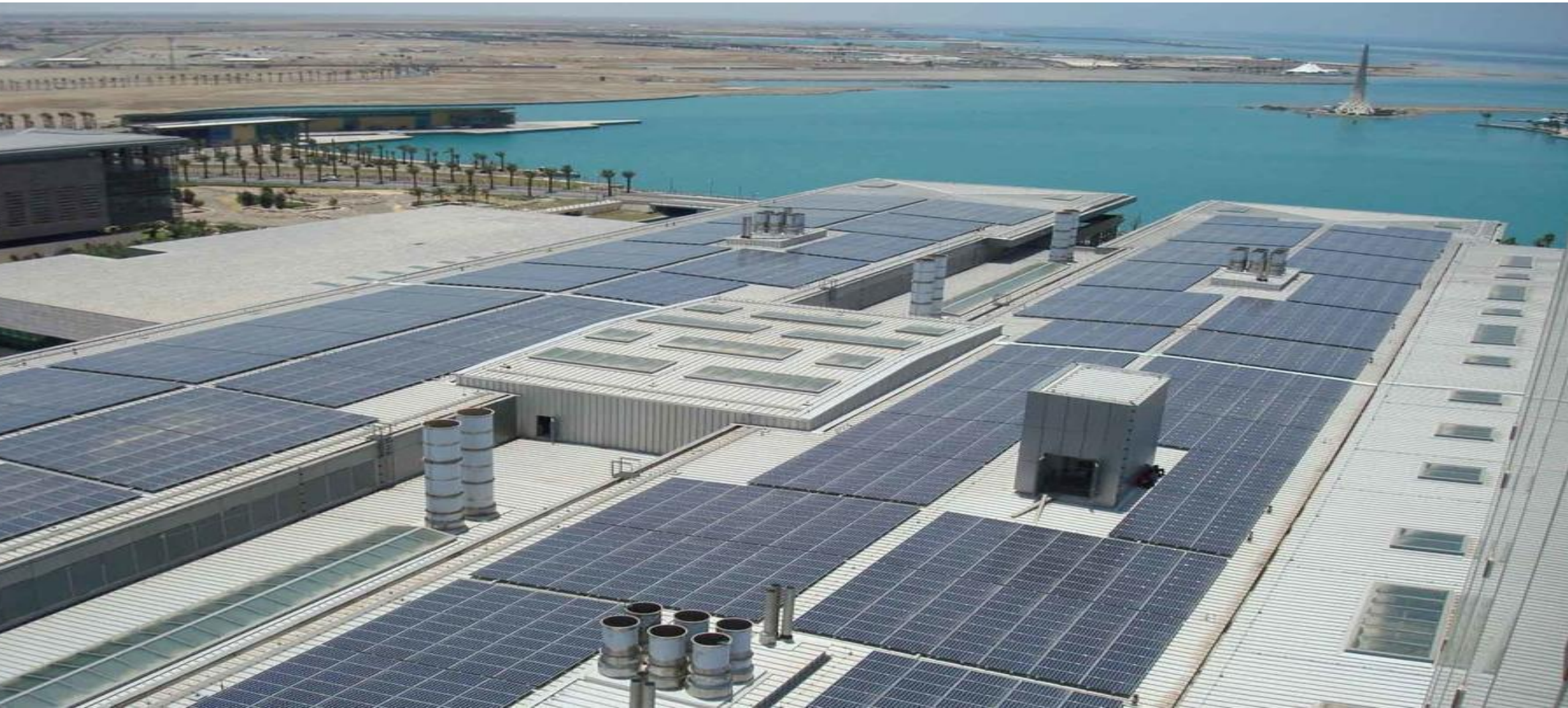
2-MW Roof-top Solar PV plant at KAUST
