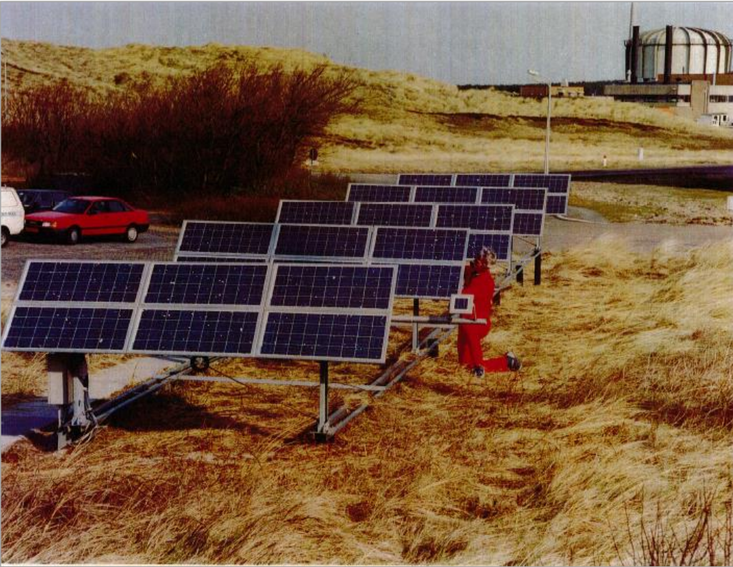
First grid-connected system in NL, ECN, Petten, 1989
