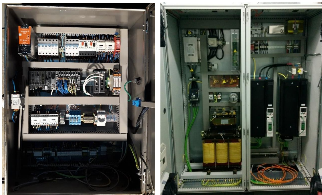
Figure 91: Back-to-back power converter and a control PLC
