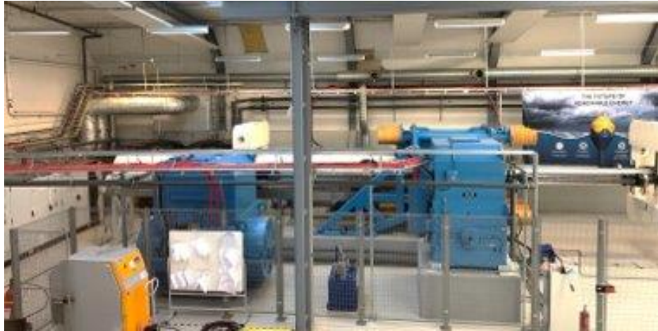
Figure 71: Images of CPO's HIL rig.
